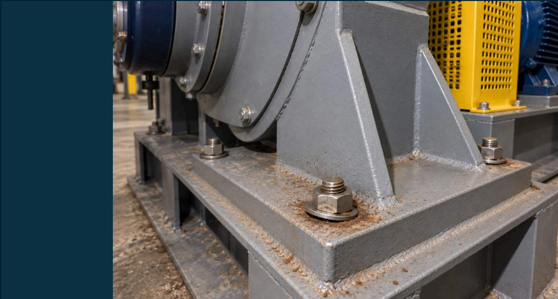
EVIDENCE 01 / Synthetic inspection photo · FAN-MNT-02
