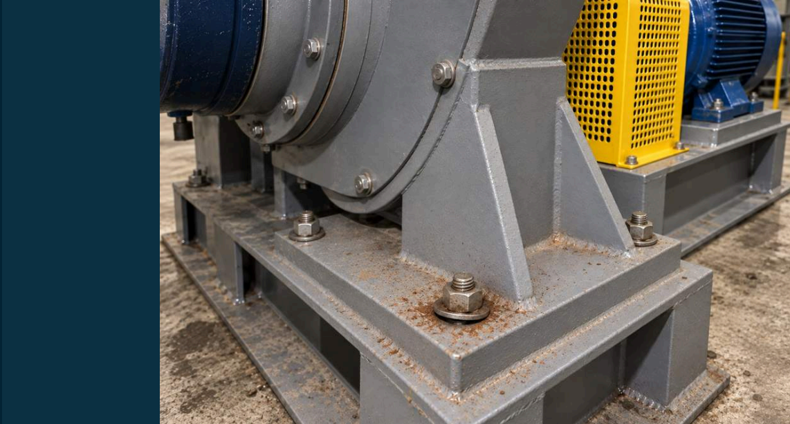
EVIDENCE 01 / Synthetic inspection photo · FAN-MNT-01
